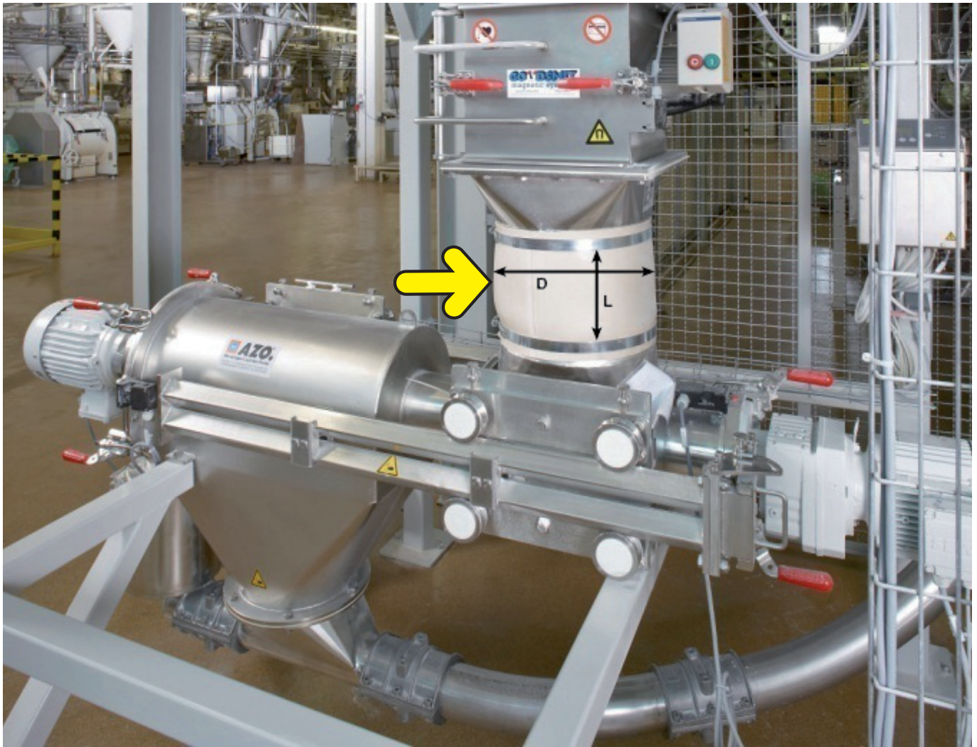
Figure 22: Compensator (arrow) in between magnet separator and sifter (Source: AZO ® GmbH + Co. KG)
