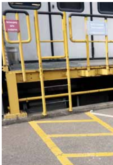
Escape routes must not be blocked
