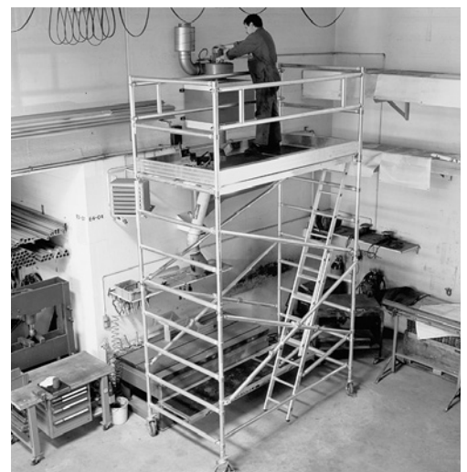
6 Missing guardrails and defective boards may cause people to fall from a height.
