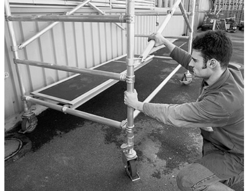
1 Fault-free mobile scaffold towers are essential for safe working.
