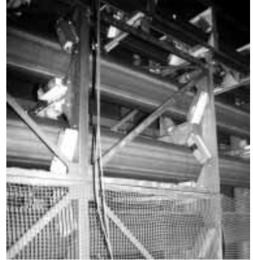
Fig. 1: Tubular belt for the transportation of spoil. Conveyor belts are often more suitable than dumper trucks.
